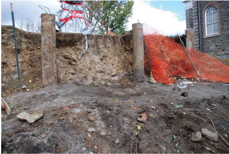
Figure 7. Profile exposed by construction contractor, disturbed grave is at base of the profile.
