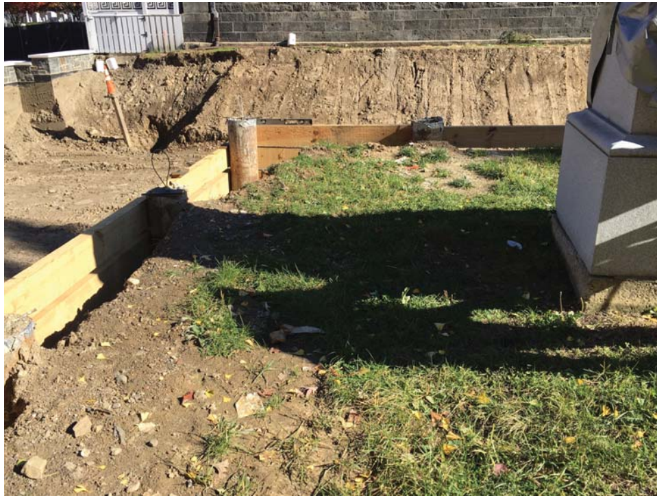
Figure 2. Ground surface at the Margaret Corbin Monument (right), showing limits of mechanical excavation at time of burial recovery (courtesy of U.S. Army Corps of Engineers).
